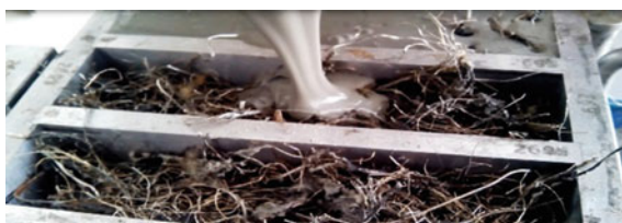
Fig. 13.20 Production of RSFRC thin panels for the shear strengthening of RC beams (Zamanzadeh et al. 2015b)
